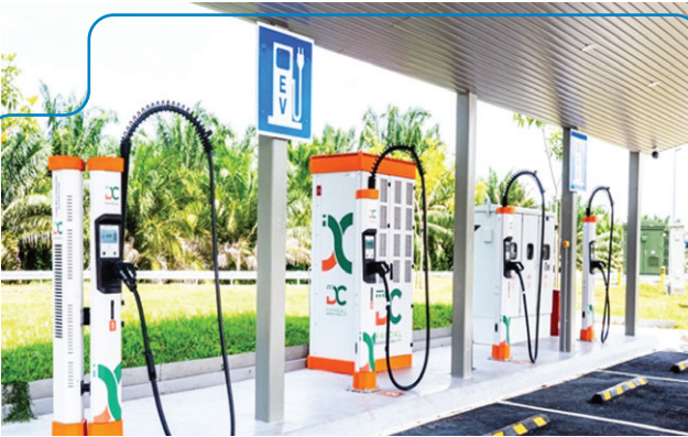
EV Charger station at certain layby
