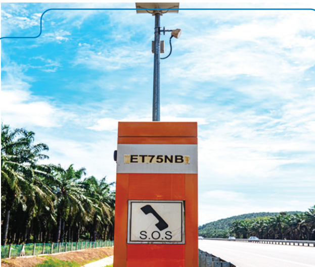
Emergency telephones on both sides of the highway at every 2 km
