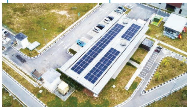
Rooftop solar panel at Kota Seri Langat Toll Plaza
