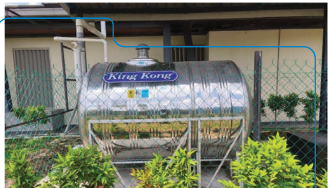
Rainwater harvester at Lekir Toll Plaza
