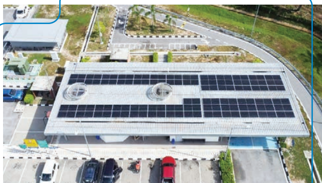
Rooftop solar panel at Assam Jawa Toll Plaza
