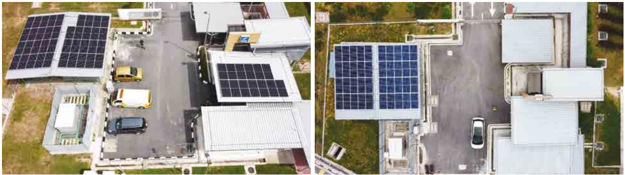
Rooftop solar panels at Hutan Melintang Toll Plaza and Kapar Toll Plaza
